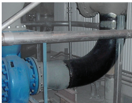
Vortab VEL installation at pump inlet
